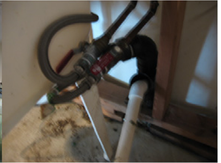
Drain out to sewer
